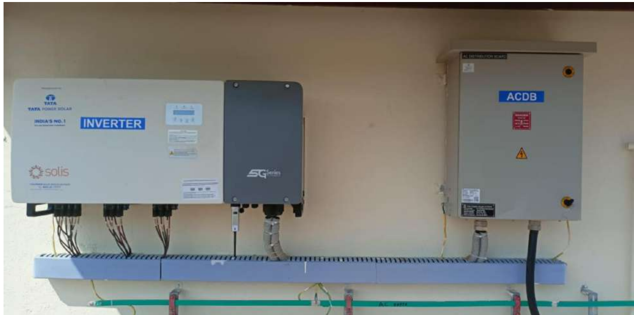
Rooftop Solar PV System Supporting Sustainable Campus Operations
